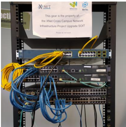
Final switch setups with LAGS
