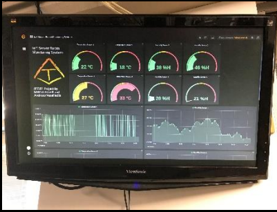
The deployed system in B203
